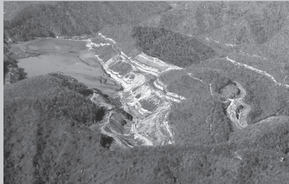
Blasting begins on the edge of the Brushy Fork sludge dam. Photo by Vivian Stockman of OVEC ( www.ohvec.org ), courtesy of Southwings flyover ( www.southwings.org ).
